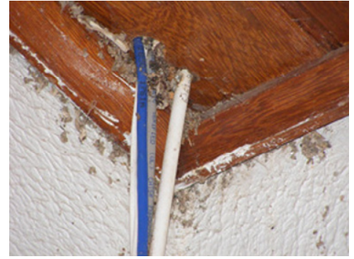
Dirt collecting in our cables
